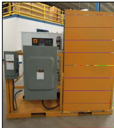
Rear View – Electrical Disconnects and Ramp
